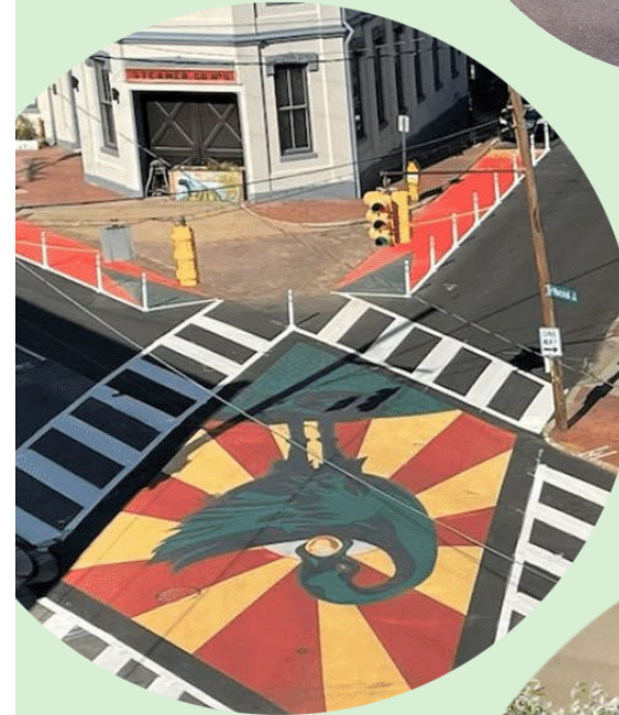
Paint can be used to make safer local streets as well as display public art.
